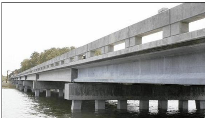
Figure 2-6: Cat Point Creek Bridge with UHPC Girders on one Span in Virginia (Ductal 2012)
