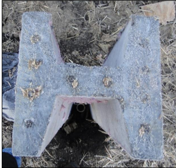
Figure 5-27: No Visible Damage on Pile P4 Head after Driving
