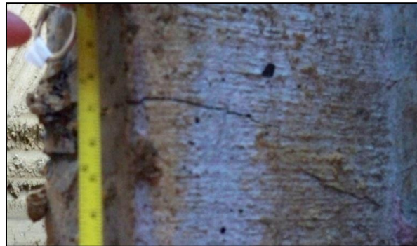
Figure 5-54: A Flexural Crack Found at a distance of 9 ft. from the Ground Surface on P4 due to the Lateral Load Test
