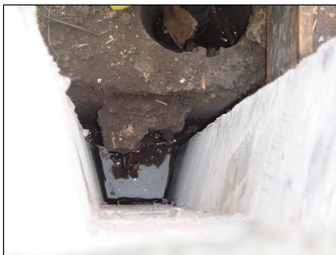
Figure 5-40: Void that Formed from Installation of P3
