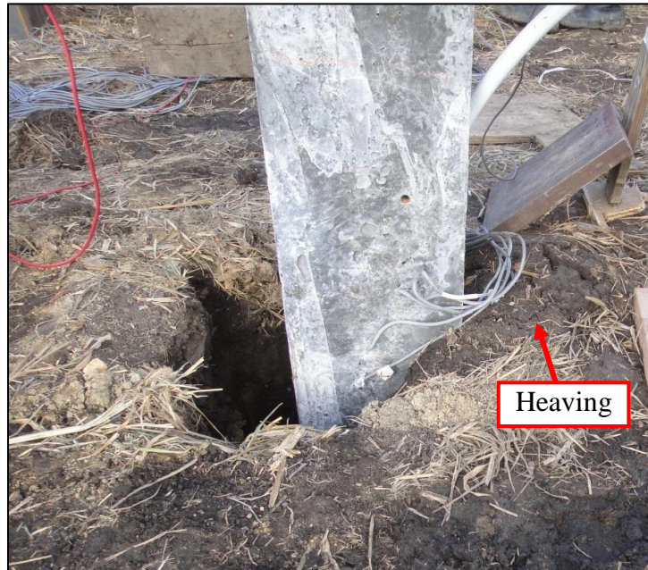
Figure 5-52: Heaving of Soil during Lateral Load Test of P4
