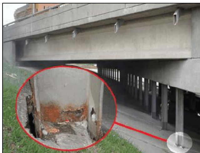
Figure 1-6: Corroded Steel H-Pile (Ehsani et al. 2012)
