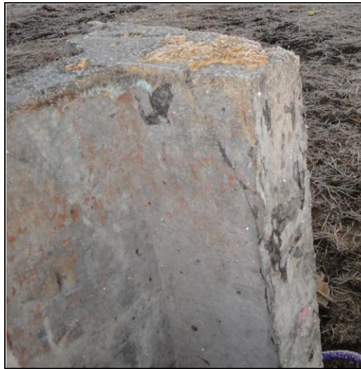
Figure 5-26: Slight Damage observed to P3 Pile Head after Driving the Pile in Place
