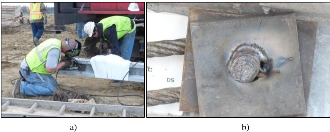
Figure 6-15: a) Welding the 2nd Washer to the Threaded Rod; and b) Pick-up Point After Welding
