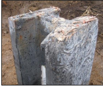
Figure 6-19: Damage to the Pile Head of UW1-2
